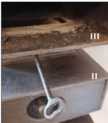
Fig. 2. The damper of the flue gas.
